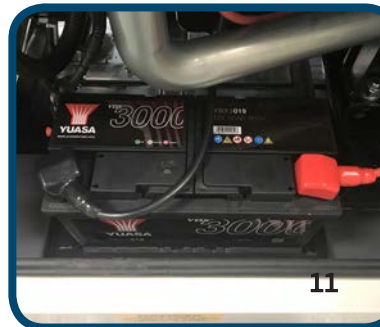
11. High quality starting battery with correct colour coded battery leads all contained in a battery containment section
