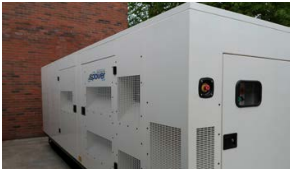
500kVA Diesel Generator
